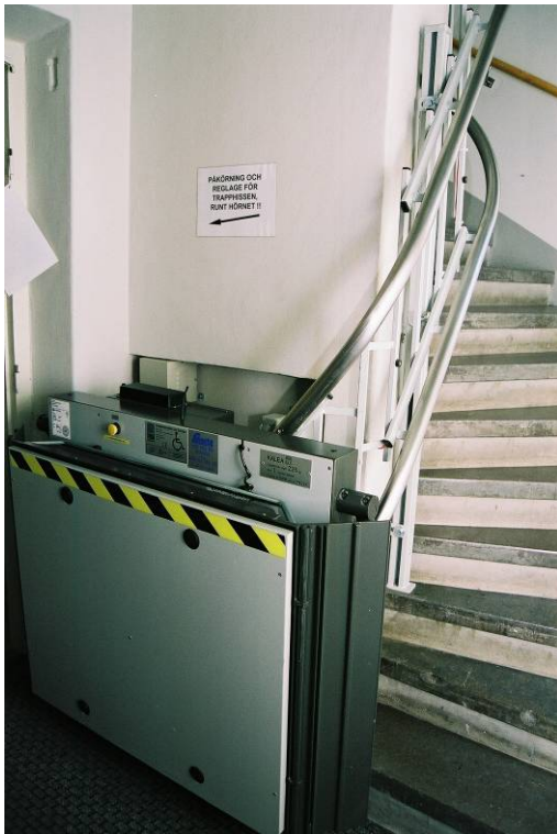
The lift platform and motor unit are installed in the vestibule on the wall next to the stairs. Jlm 05m212/13
